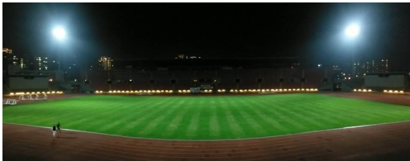
Field demonstration to replace HID lamps with ultra-high-power LED lights saves 50% of electricity
