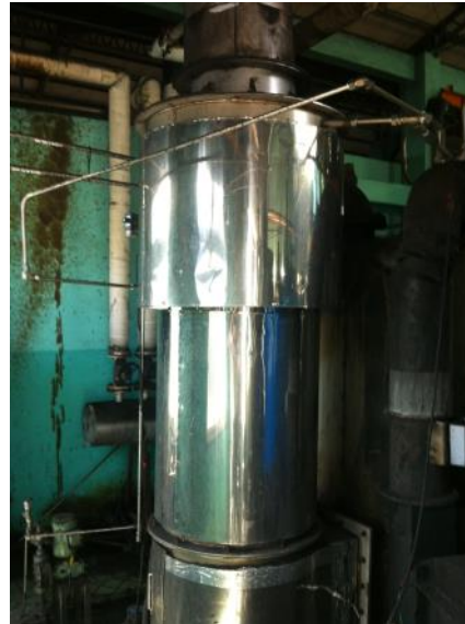
Hydrogen-enhanced combustion system for boiler
