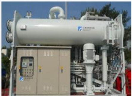
petrochemical 200kW screw-expander low-temperature ORC power generation system
