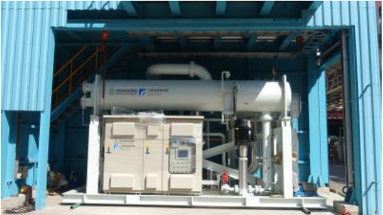
iron&steel 200kW screw-expander flue gas ORC power generation system
