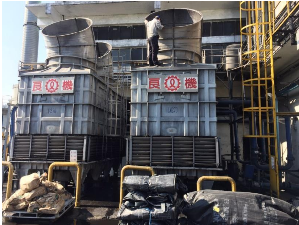
Cooling towers are integrated
