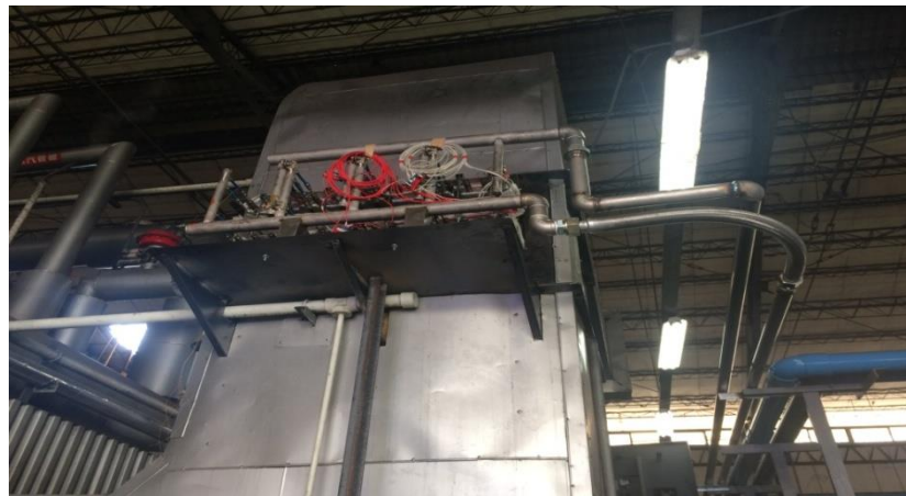
Smoke recovery 2KW power generation
