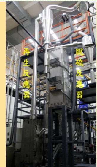
Warm/Hot Gas Cleaning
