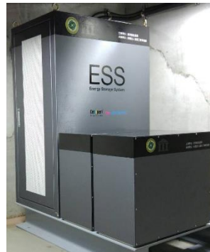
Energy Storage System in NSYSU
