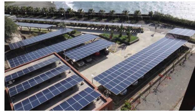
Solar Panel Parking Lot
