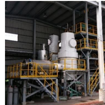
5 t/d paper-reject pyrolysis system
