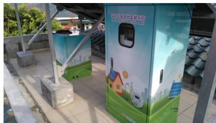
PV, ESS, and Fuel Cell Based Microgrid in Shenzhen
